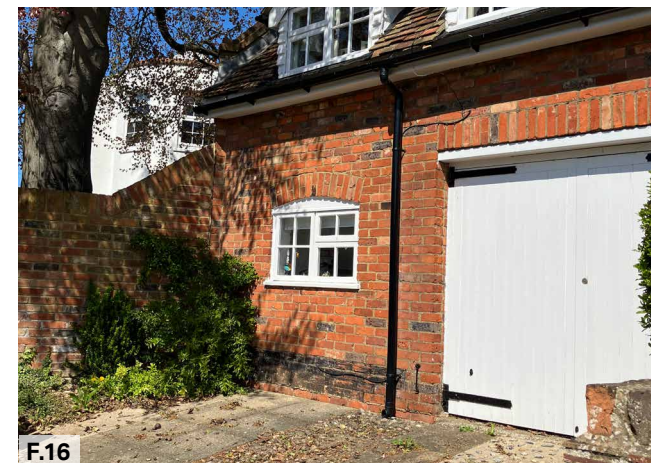
Figure 16: A garage structure constructed with traditional materials that respect the local vernacular
